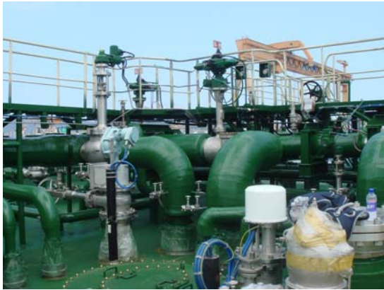
Figure 1 Photo of the valves are installed on vessels
