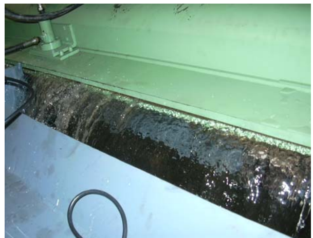
Figure.9 Water curtain cooling system
